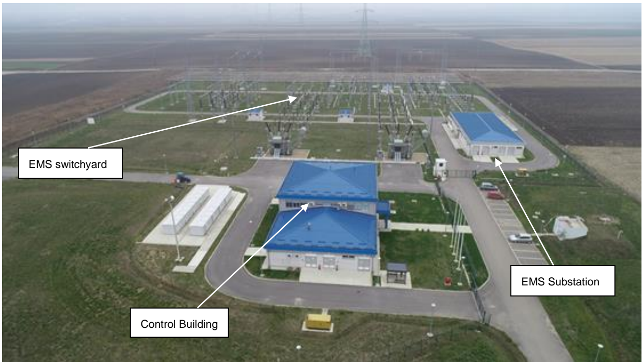
Figure 5-1 Čibuk Control Building and Electrical Compound
