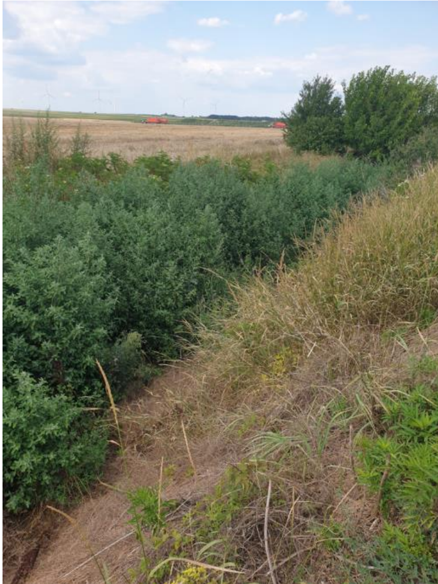
Figure 2-5 Drainage ditch with scrub growth
